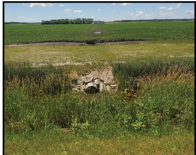
Side Water Inlet with 5 ft Buffer
